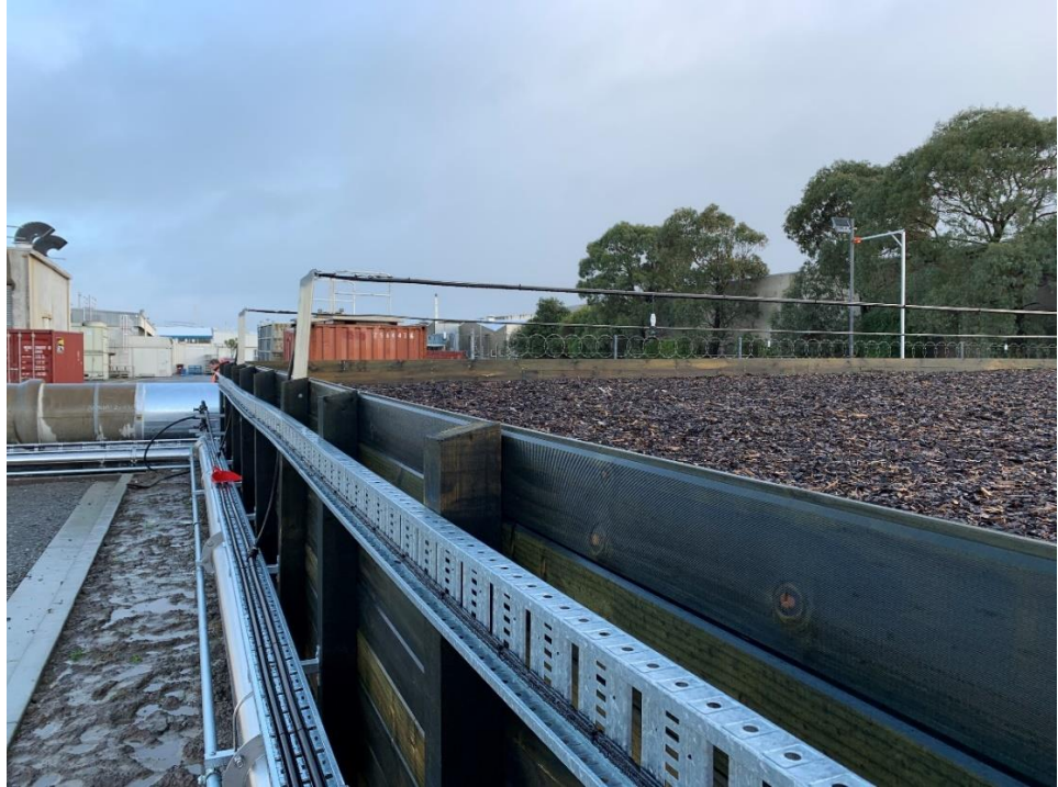
Figure 1: Photograph of Tegel Biofilter (7 July 2020).
