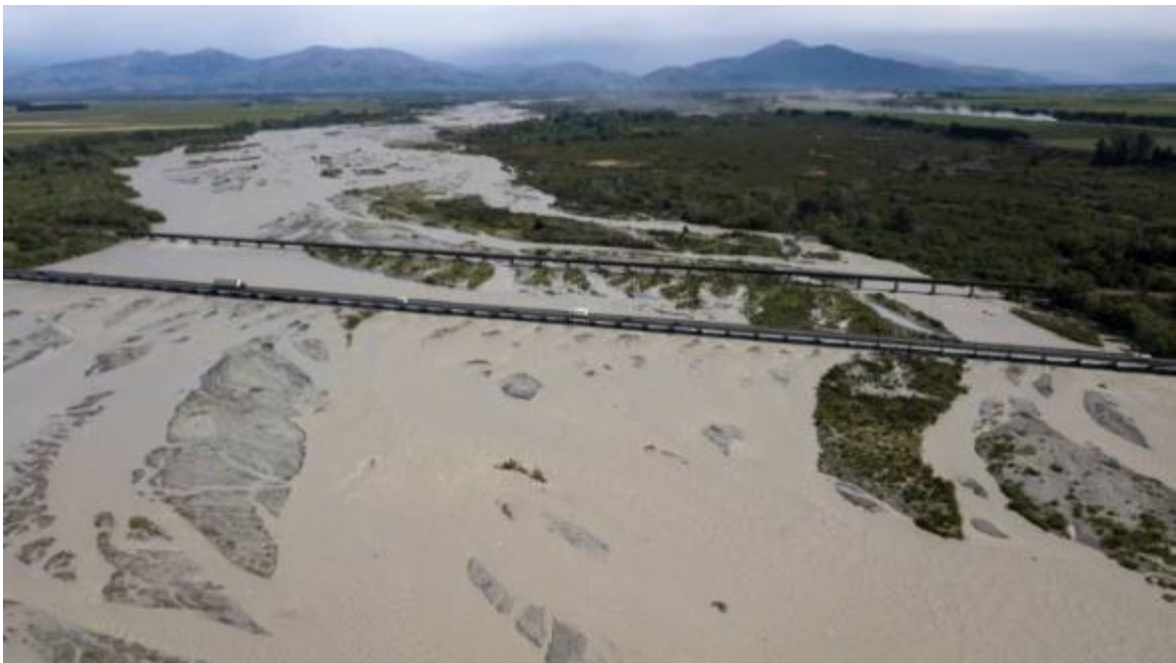
Fig 6. Rangitata river SH1 bridge December 2019 (photo: stuff.co.nz)
