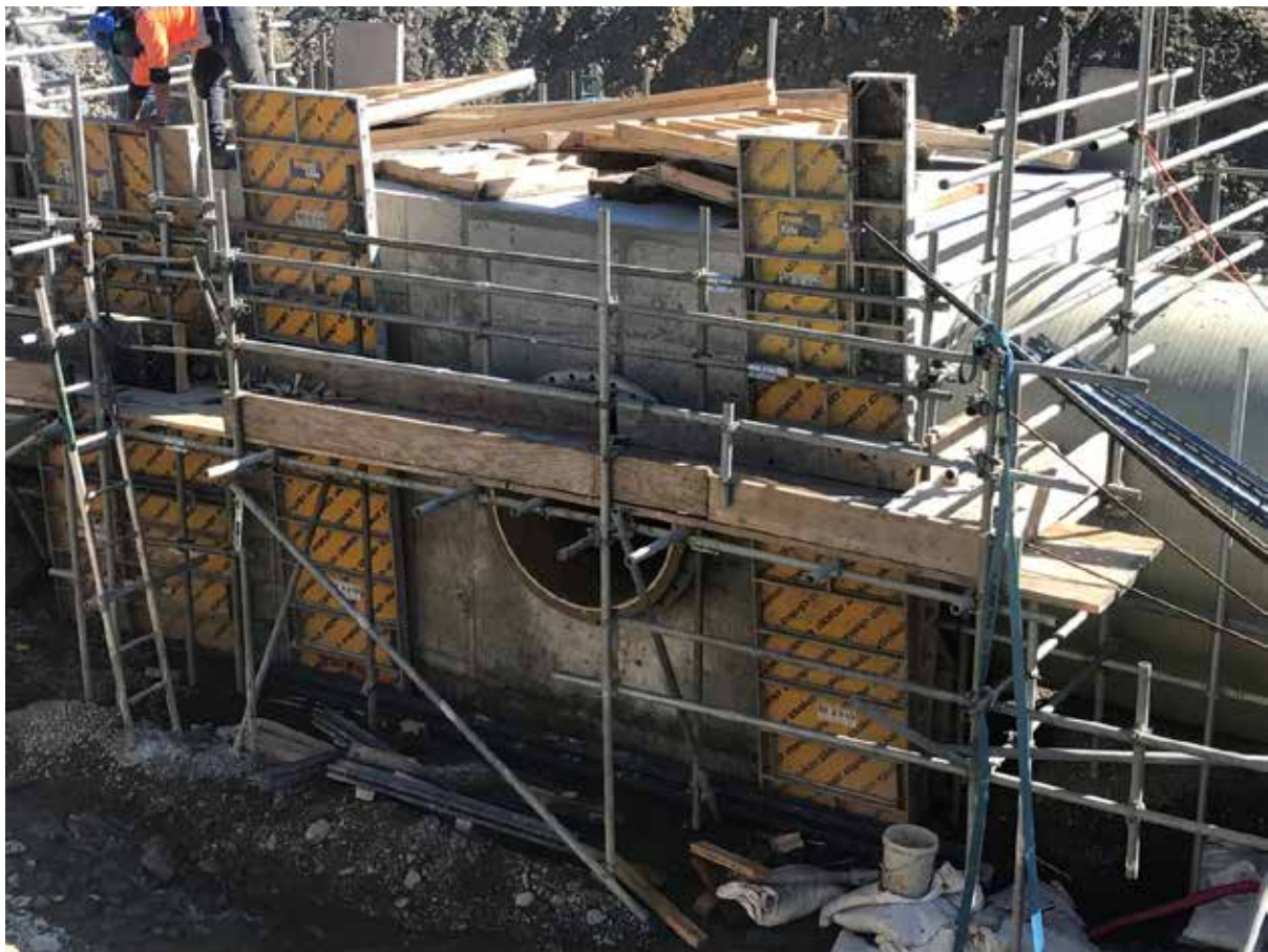
Figure 7. Selwyn/Waikirikiriri Near River Recharge (NRR) Project offtake
