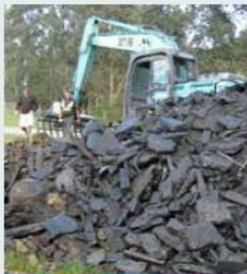
Evidence of the illegal dumping of earthquake demolition waste
