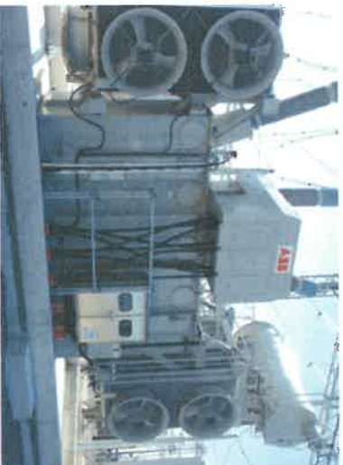
Islington 220/11kV Transformer T1
