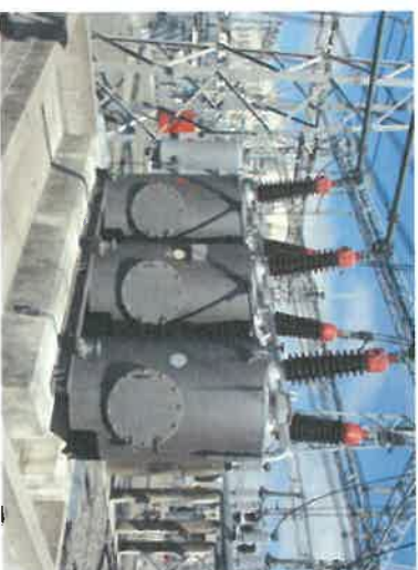
Islington 66kV Oil Circuit Breaker T12
